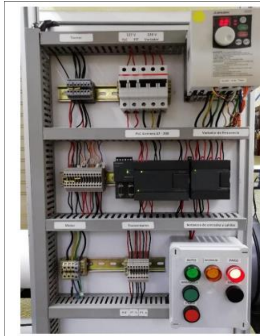
Figura 2-10 Gabinete de control [13].
