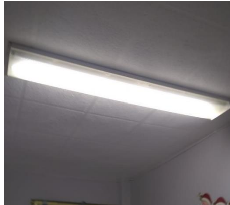
Figura 3.7 Luminaria fluorescente instalada
