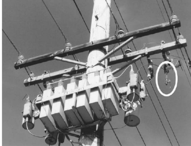
Figura 2.14 Banco capacitor con un fusible abierto. (Copyright © 2002. Electric Power Research Institute. 1001691. Improved Reliability of Switched Capacitor Banks and Capacitor Technology.)
